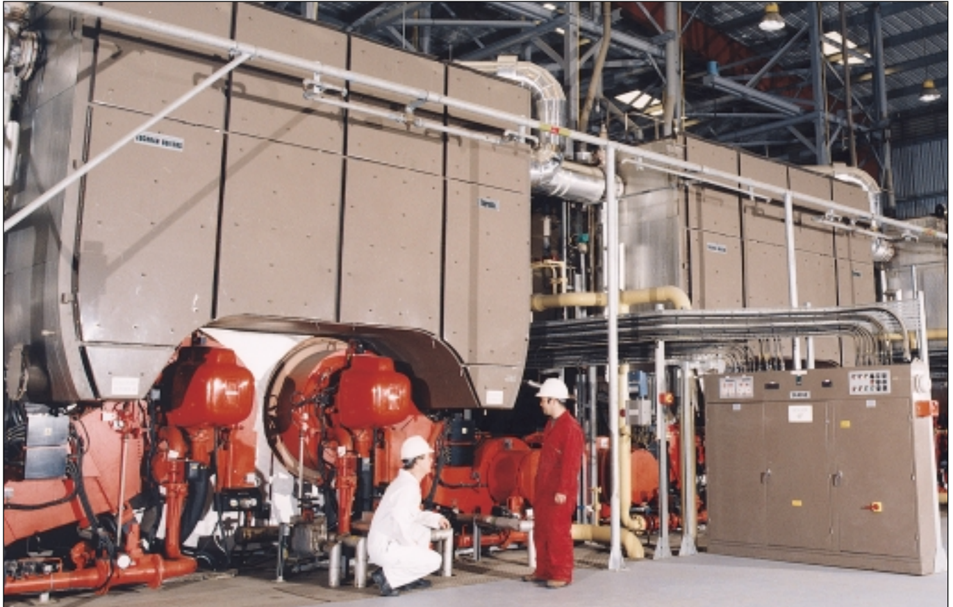
BIB Cochran 6x 32 Tonne per hour Steam Boiler CHP Installation
