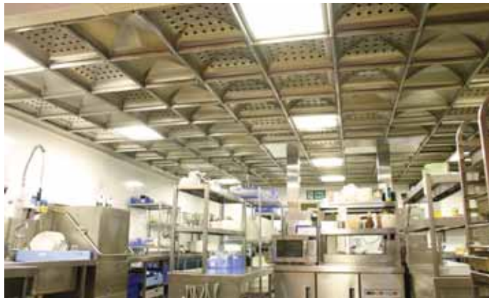
Heydal ventilated ceiling at Sandy Balls holiday centre in the New Forest
