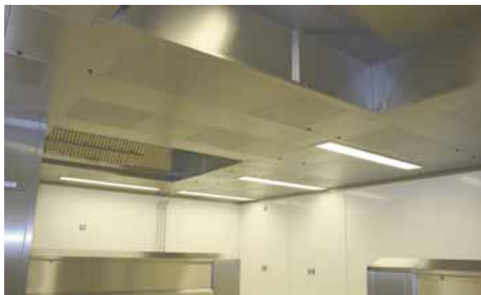
Silverline ventilated ceiling system at Garth Prison in Lancashire
