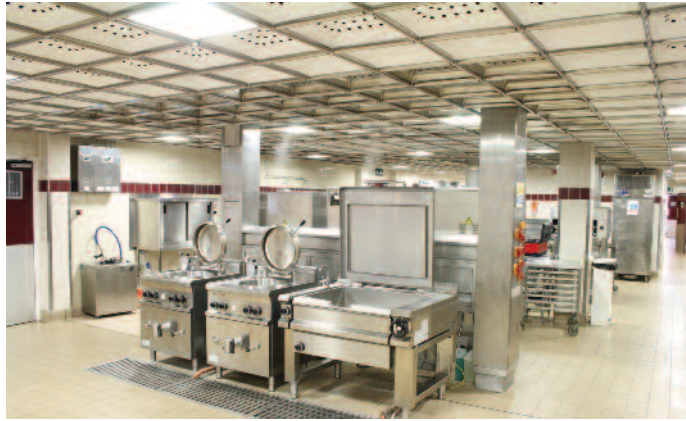
Heydal ventilated ceiling at Fort Blockhouse in Portsmouth
