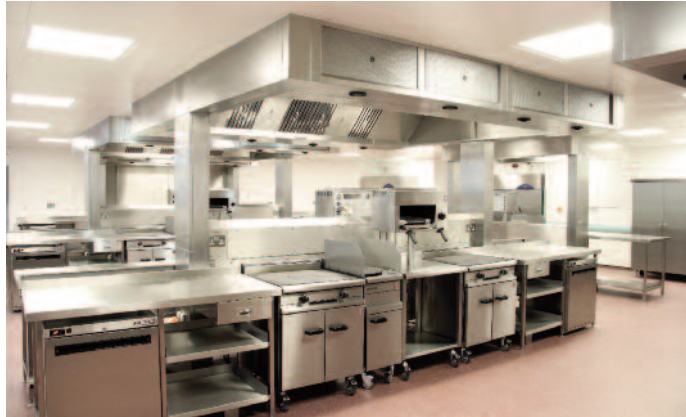
One of 84 Ultrastream UV canopies installed at DFSS Worthy Down
