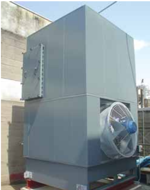
Forced draught counterflow tower with cooling airflow being provided by a low level side mounted directly driven axial fanset
