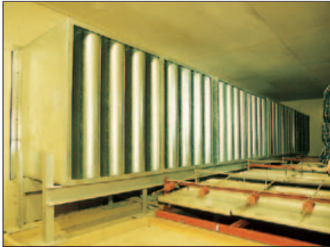
EMTEC RAAC silencers attenuate a plantroom discharge
