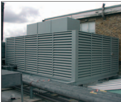
EMTEC LAAC 15 acoustic louvred screen around chillers
